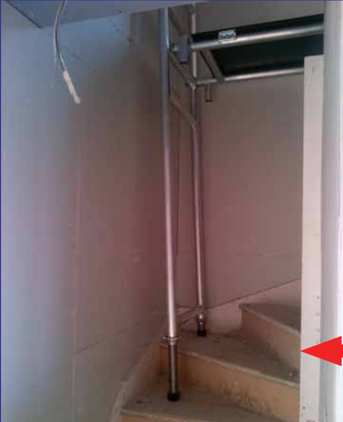
Stairsafe frame supports kitewinder platform at lower end of stairs
